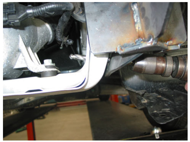
Figure 6: Drill hole in radiator support using steel mounting bracket as a guide.
